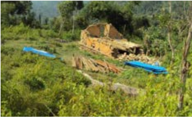
Photo 9: House damaged due to shifting of land by 4m in Aureniby due to land displacement
