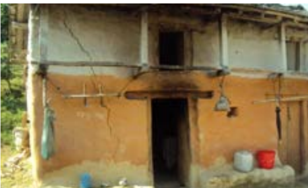
Photo 4: Cracks developed in the house in Balaucha
