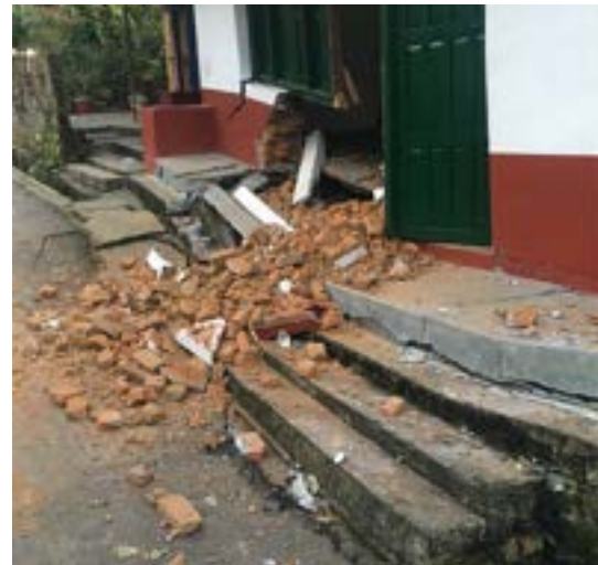
Figure 12: Damaged of house due to subsidence of land in Kushma Bazar:
