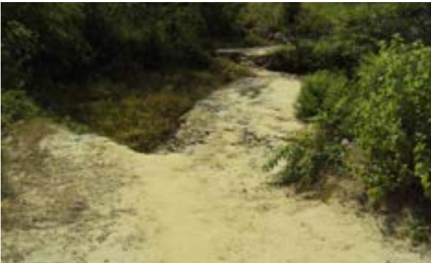
Photo 2: Shifting displacement of existing motor-able road by 4m and slide 2m down
