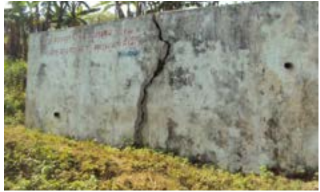
Photo 5: Cracks in the public water tank
