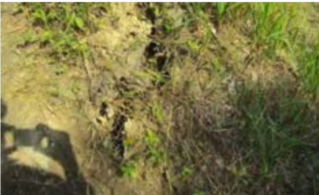
Photo 3: Cracks on the Hillslope
