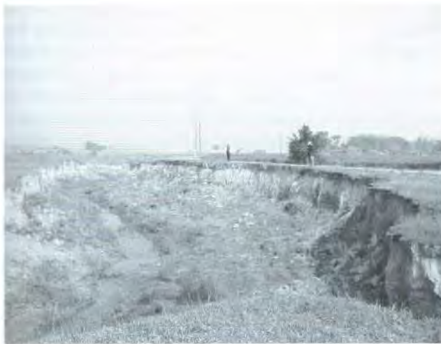
Fig. 10. Bank erosion in Dhanpura Khadara Village.
