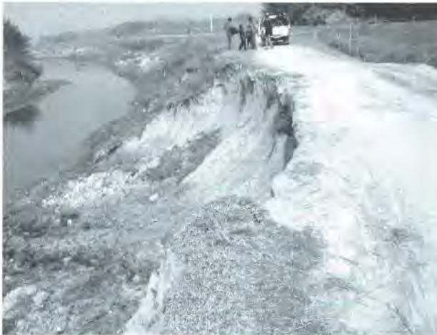
Fig. 8. A typical example of riverbank failure
