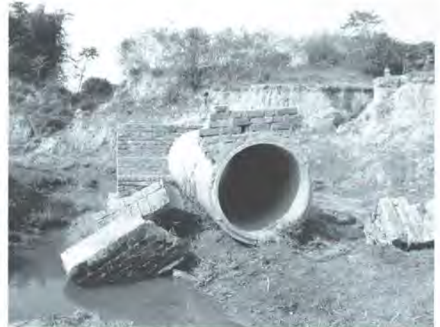
Fig. 9. Collapse structures found in the nala which was collapsed during the construction phase.
