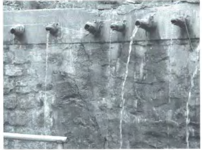
Fig. 8. Close view of 108 holy spouts located behind the Muktinath Temple and diagonal cracks in the wall
