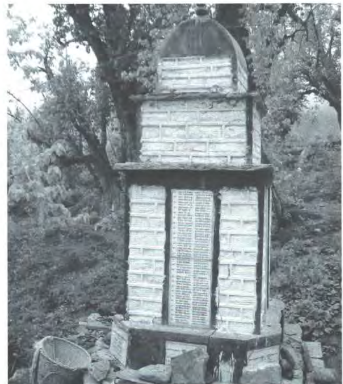
Fig. 10. Damaged monument due to ground settlement located in front of the Muktinath Temple.
