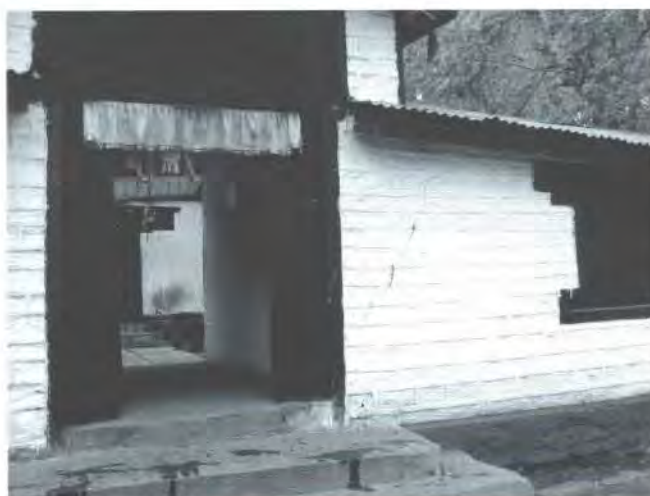
Fig. 9. Few mm. wide diagonal crack in the wall of the first entrance of Muktinath Temple.
