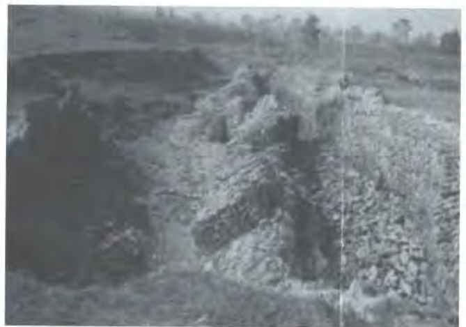
Fig. 8. Failure of gabion wall in the west of Khuniyakatta village (Lakhantari VDC) constructed to divert irrigation water into Singhiya Khola.
