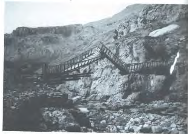
Fig. 15: Up-bulged wooden bridge of Jhon Khola due to creeping
