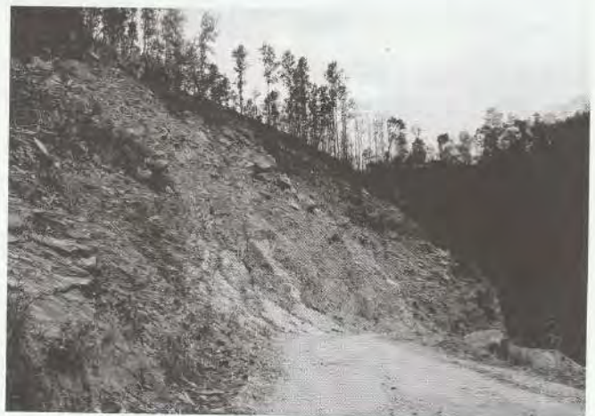
Photo: 6 Manmade causes of landslides in highly fractured quartzite on Gurung Sera-Patchaur road due to construction of road by disturbing natural slope
