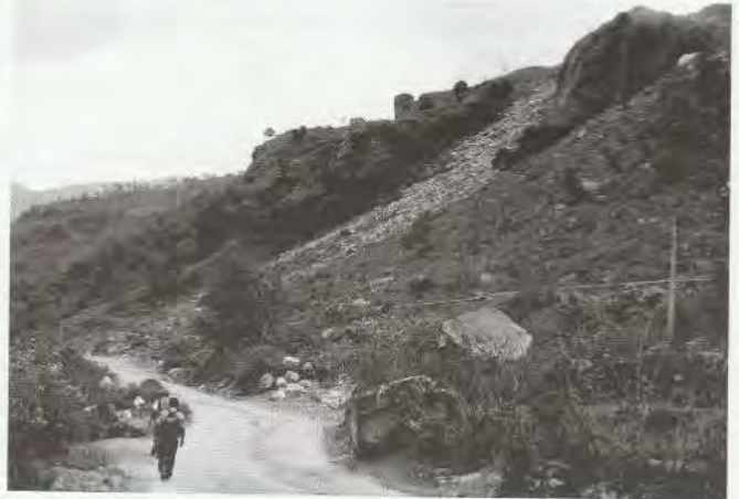
Photo: 2 Highly disturbed hill slope on the way to Galeshwor from Beni Bazaar
