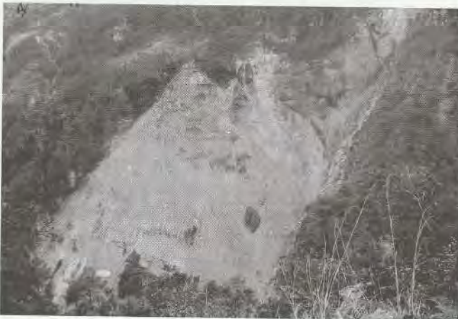
Photo: 3 Huge landslide at right abutment of the Raughat Khola just downstream of Tatopani below Thirbang village
