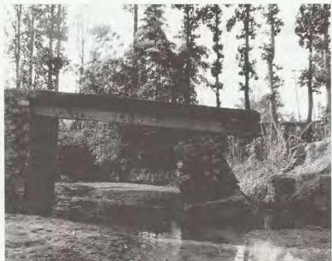
Photo 14 Collapse of bridge at Bame Khola. Poor construction material and weak anchoring led to foundation failure.
