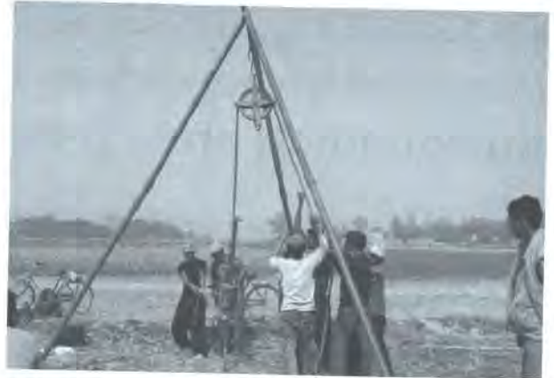
Photo 2: Preparing for Standard Penetration Test (SPT) to understand bearing capacity of the soil
