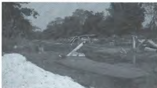
Photo 7: Remaining of 2 foundation pillar out of 5 in the bridge at Daduwa Khola near Kuniya, Manikapur-3
