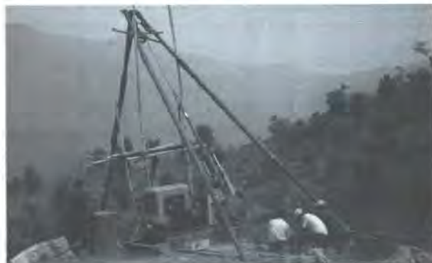
Fig.5: DDH-2, Drilling assembly, Acker Drill machine, Lister engine Boyles Pump, Hoisting engine, Tripod, hoist and pulley, drilling rods, core barrel, core catcher, casing rods etc
