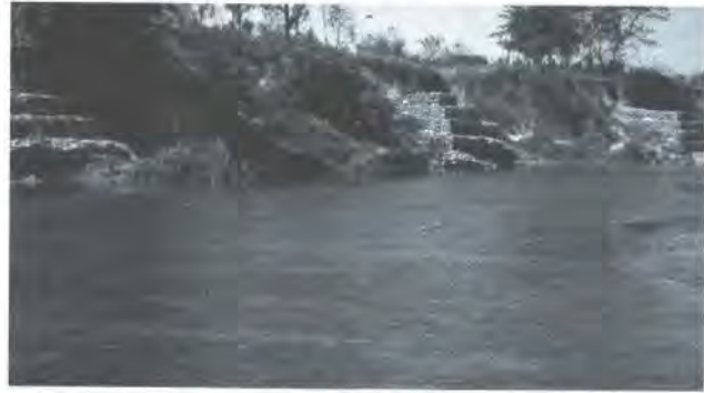
Photo 3: Spurs constructed in the south of Kunia village in the Daduwa Nadi to control bank cutting but their repair and maintenance is poor
