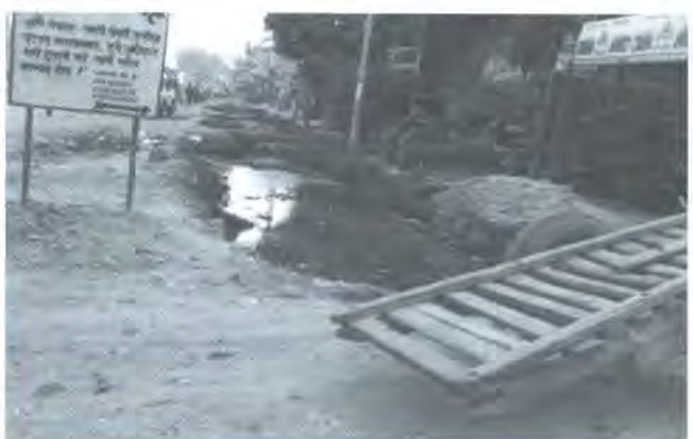
Photo 9: Drain not completed in the road near teaching Hospital
