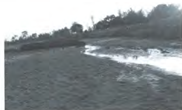
Fig. 14: Washed away of gabion spur in the Jaladh Khola
