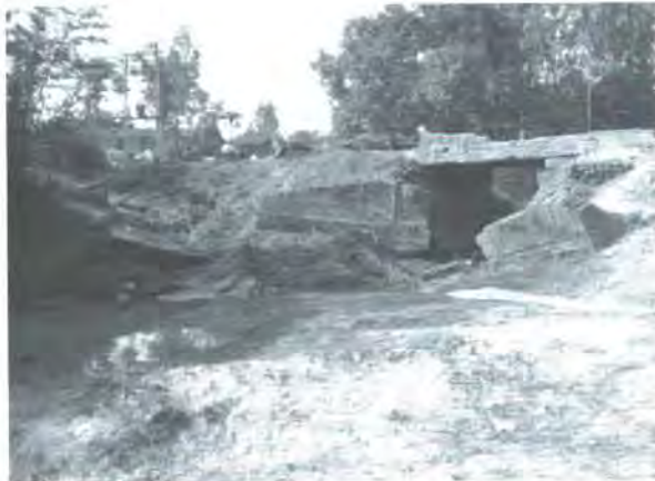
Fig. 15: Damaged Bridge due to the high flow of water in 2008
