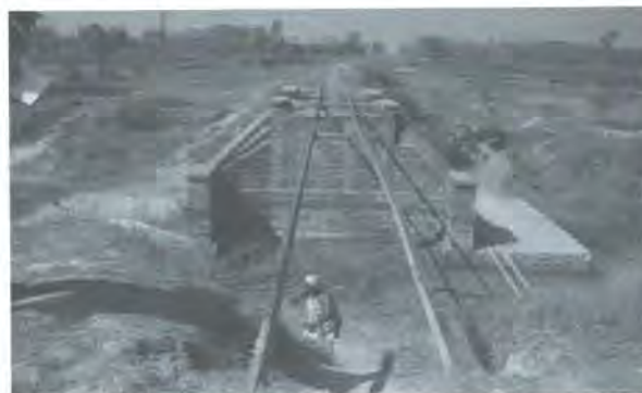
Fig.16: Damaged railway awaiting its repair and maintenance line in NW of Janakpur Cigarette Factory
