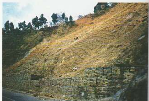
Bio-engineering activities to stabilize the landslide along the Amiko highway at 61.7km.
