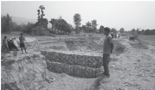
Fig. 17: Soil erosion taking place near the Kathepul due to construction of road which clogged the drainage system and construction of the gabion wall at the same place.
