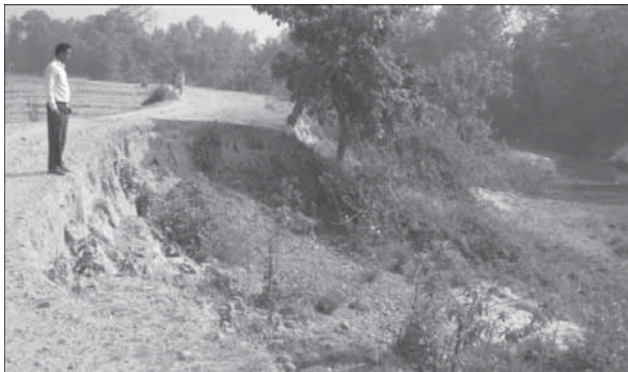
Fig. 16: Road constructed along the right bank of the BhasiKhola, near Bhasigaon was eroded. No preventive measure has been taken.
