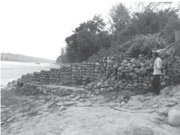
Fig. 13: Washing away of gabion spur in the Narayani River.
