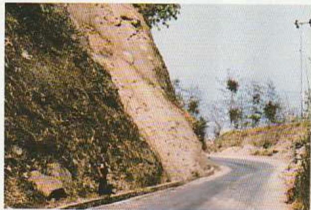
Photo 23: Landslide reactivated by steep slope cutting.
