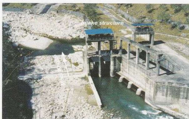
Photo 6: Water of the Modi Khola diverted to the tunnel on right side of the river in Intake site of Modi Khola power house
