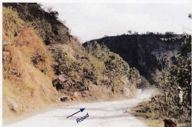
Photo 13: Landslide debris occupying the road at Bayerbot.
