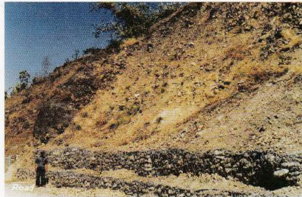
Photo 21: Landslide affecting the road south of Beni.
