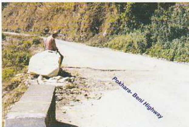
Photo 8: Fall of the ripple marked quartzite, which has damaged the road.
