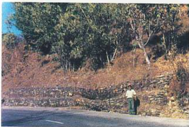
Photo 22: Bulging gabion wall due to soil creep.
