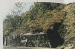
Soil Creep pushing out the protection wall.
