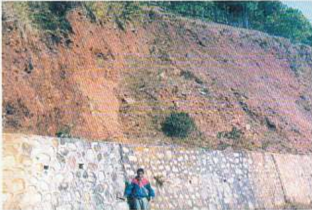
Photo 26: Landslide with protection wall at the toe of the slide.
